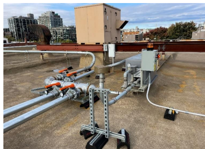
Example of a commercial SVI installation on a Brooklyn rooftop
